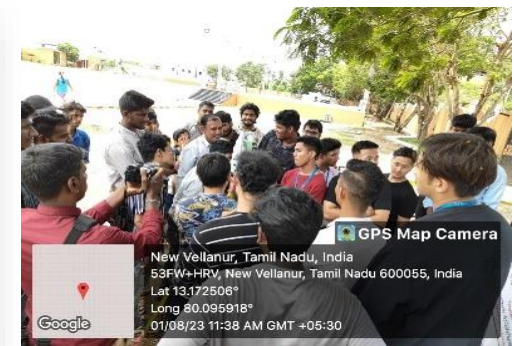
Foundation marking and layout preparation for buildings Mr. Selvaraj, Managing Director, Athira Geo Spatial Services Private Limited, Chennai
